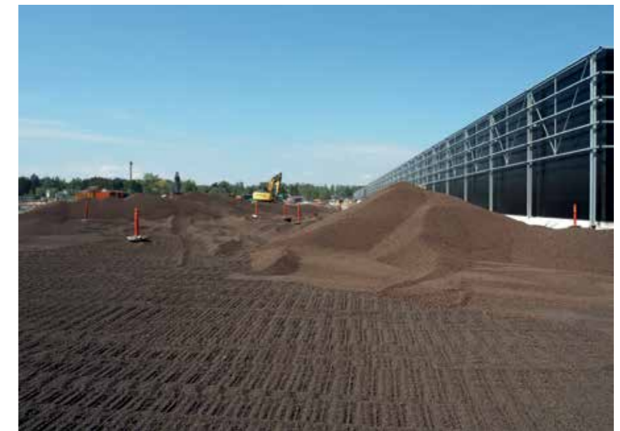
The thickness of the Leca lightweight fill layer in the structure of the yard varies between 300 and 1,200 mm.
