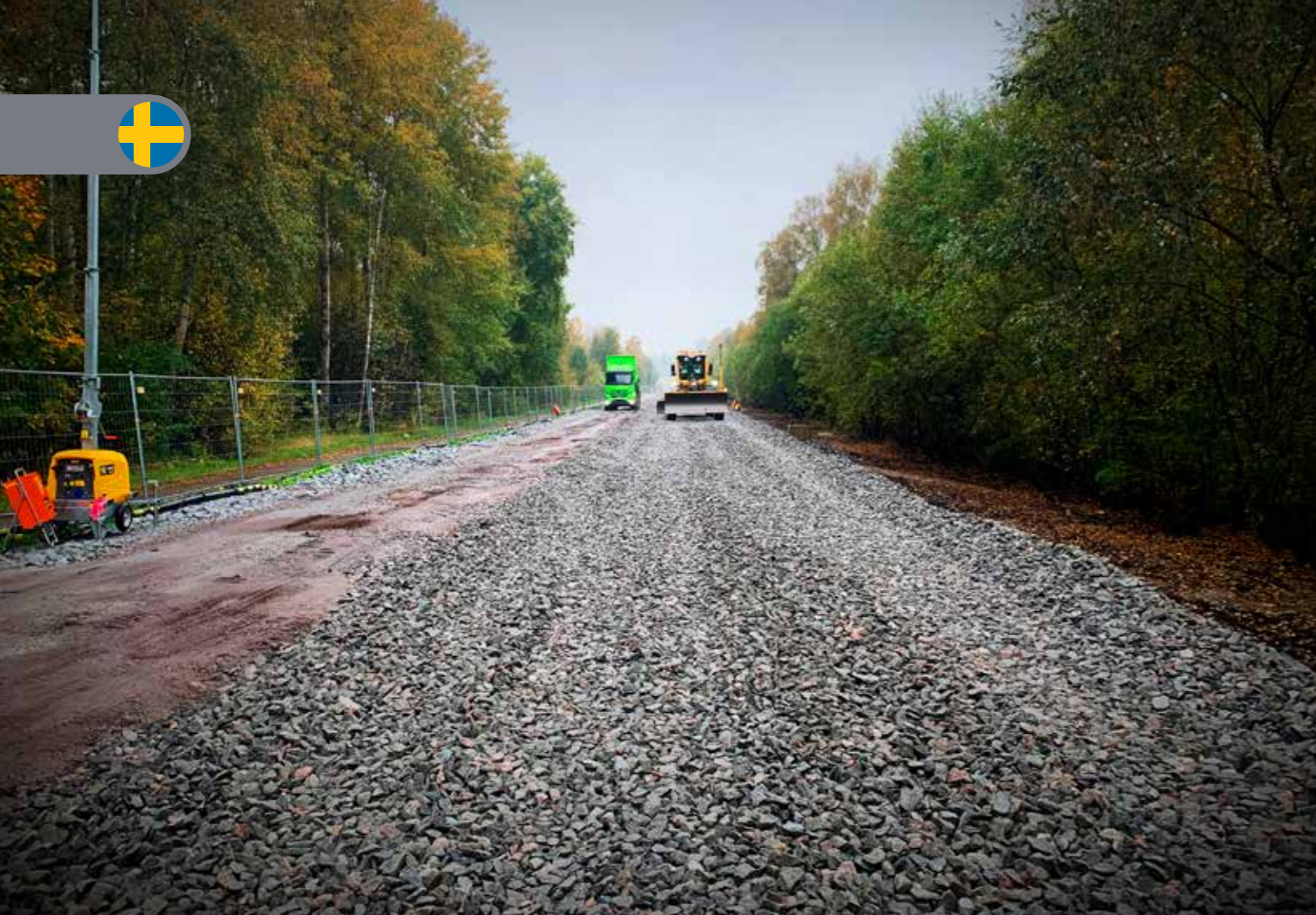
On top of the finalized Leca solution crushed stone was placed before installing the new railway tracks.
