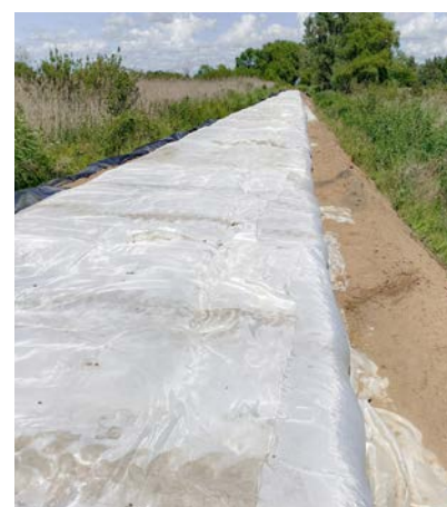
Structural fill in the form of “mattresses” made of lightweight expanded clay aggregate wrapped in geosynthetic fabric
