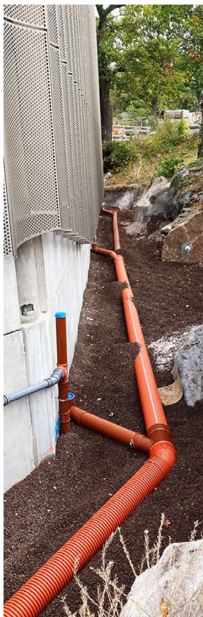
Leca LWA is used as backfill to stabilize the porous rock next to the building.
