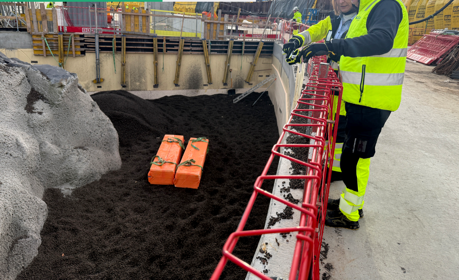
Representatives from Leca visiting the project site to inspect the installation of Leca® LWA, used to reduce earth pressure and improve safety and efficiency in a confined construction area.
