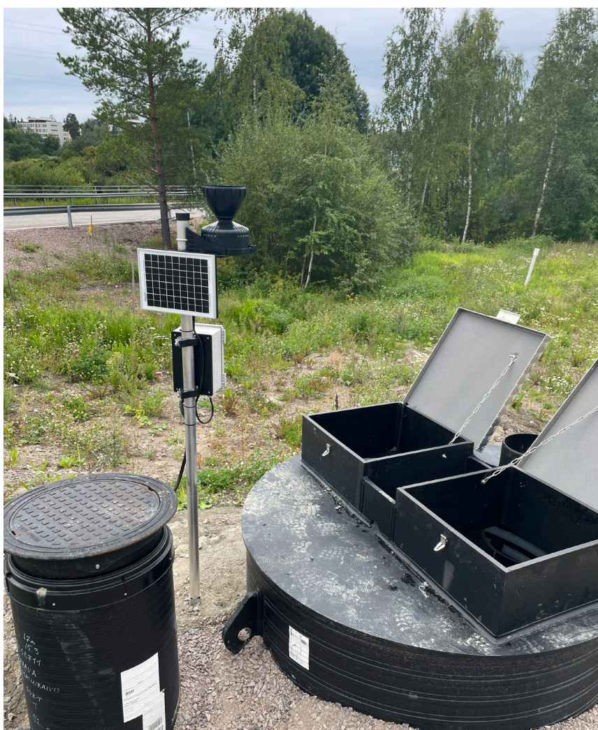
Filter chamber combines sedimentation and Filtralite P filtration.
