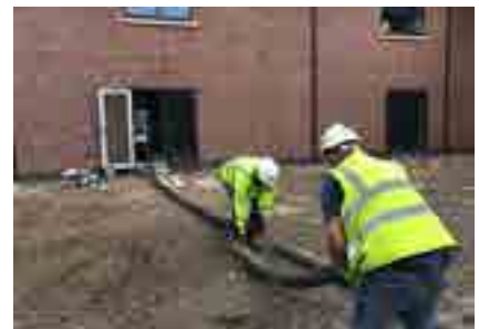
Crushed rock aggregate would have posed a serious risk.
