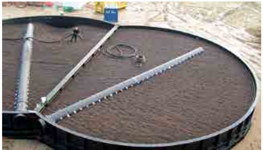
Filling of the odour treatment filter. The pipes on top are the outlet of the cleaned air.
