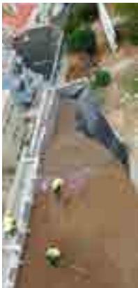
The gap between the new wall and the existing slope was filled with Geo Leca.
