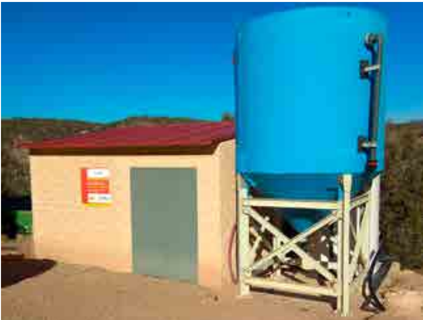
View of the small plant with the sedimentation tank outside.
