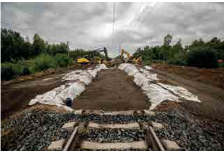
The railway track between Kokemäki and Rauma in Finland was repaired using Leca Lightweight Aggregate filling.
