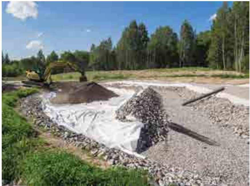
The other section contains crushed (grain size 3–8 mm) Leca LWA manufactured in the Kuusankoski factory of Leca Finland.
