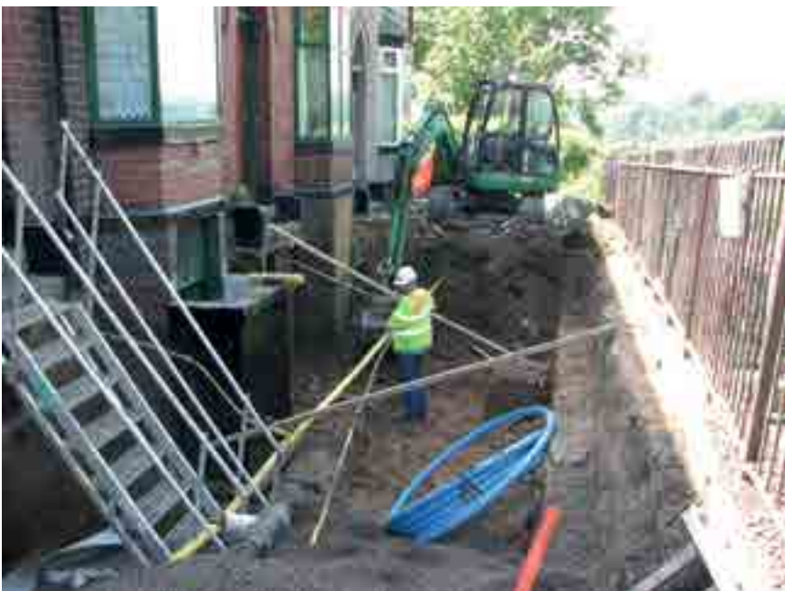
Leca LWA was found to be the ideal material to replace the traditional backfill
