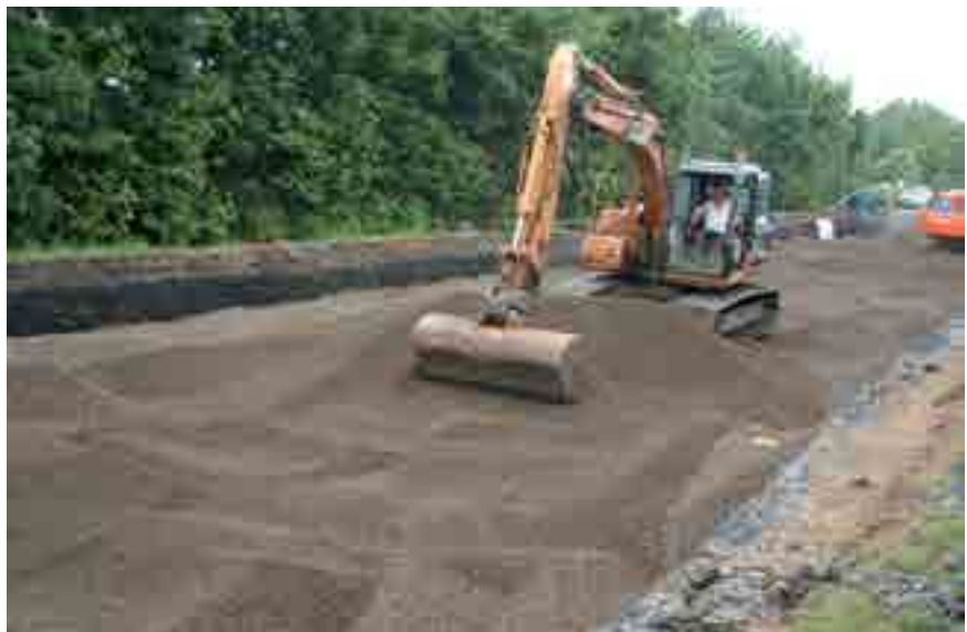
The strength and compaction properties of Leca LWA provided an opportunity for heavy vehicles to continue the installation process.
