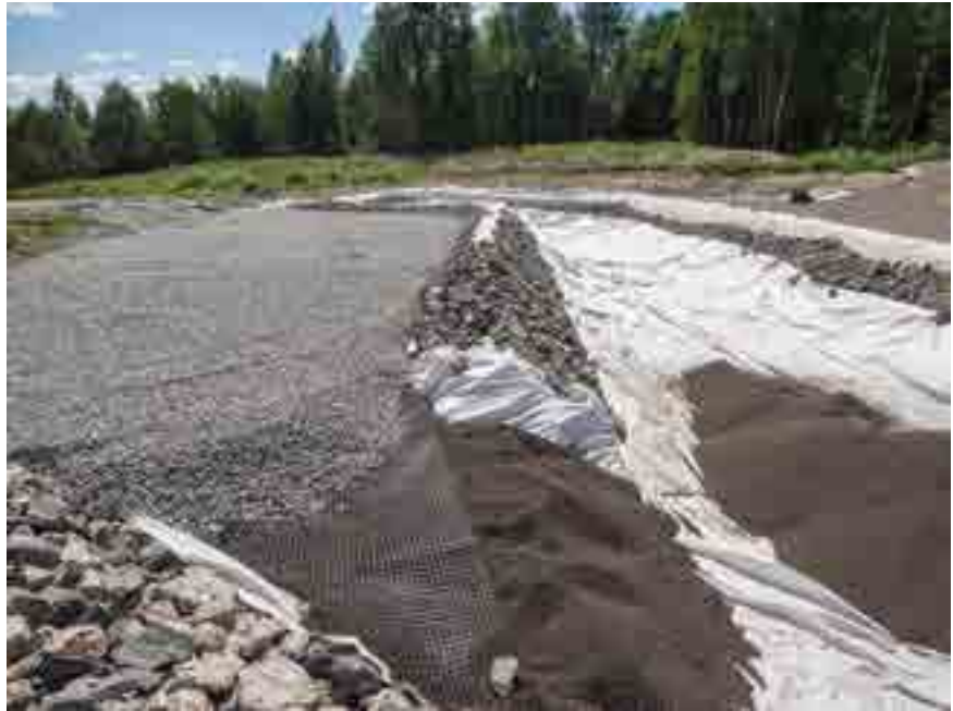
One section contains more fine-grained Filtralite P filtration material that is produced at the Leca factory in Raelingen, Norway.
