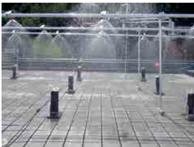
Klima 2050 focuses on solutions with high water detention capacity and are able to run extreme test. Here water detention of permeable pavers with a Leca sub-layer is tested. Photo: Tore Kvande, NTNU
