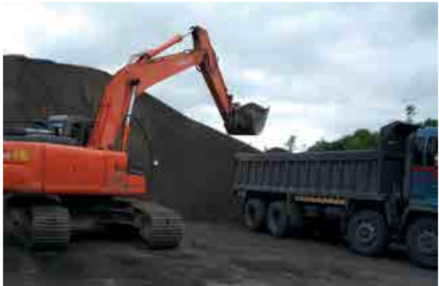
Over 5000m³ of Leca LWA was used to complete this ambitious project.
