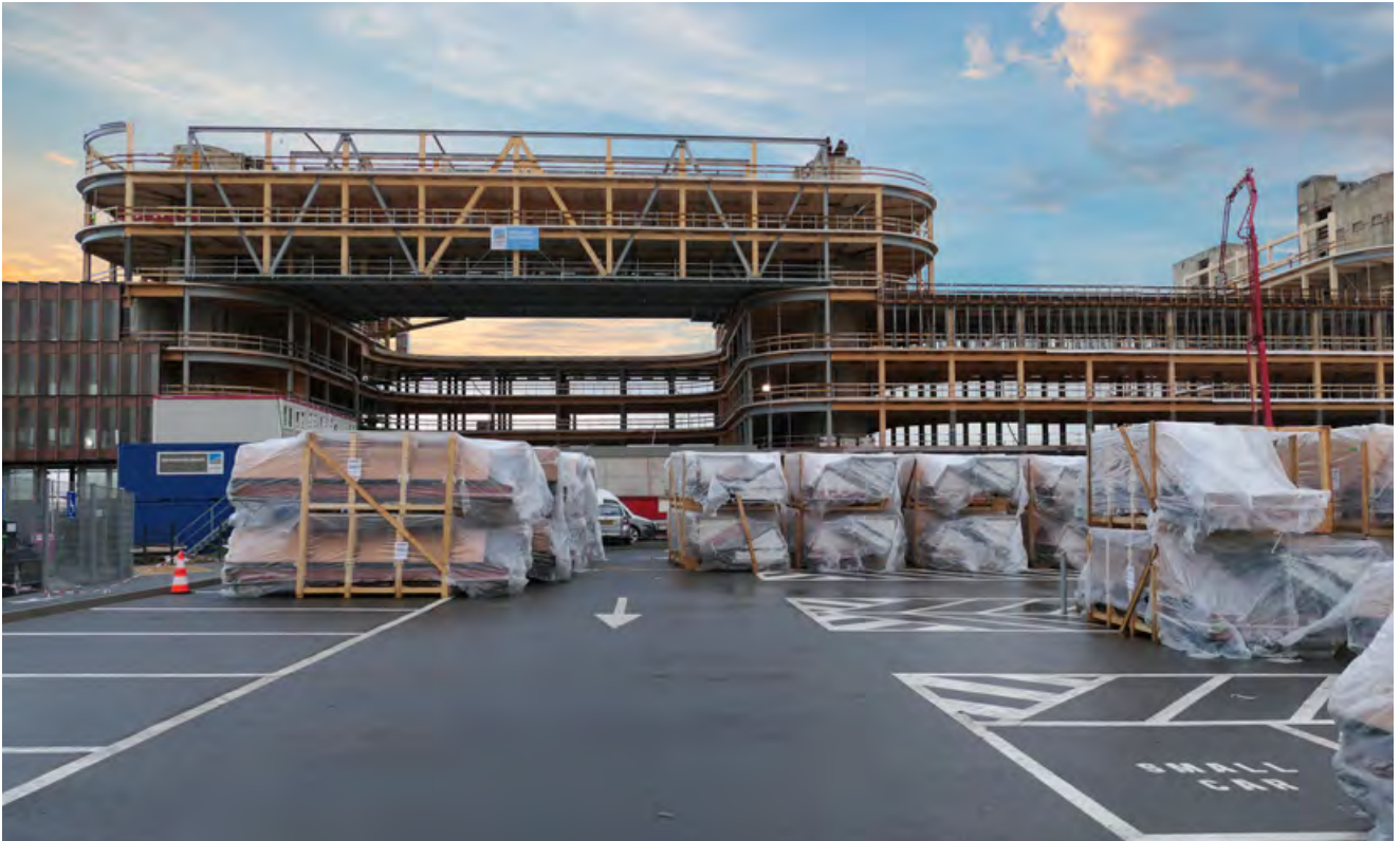
The Skypark Business Centre at Luxembourg's Aitport is currently the largest timber construction in Europe
