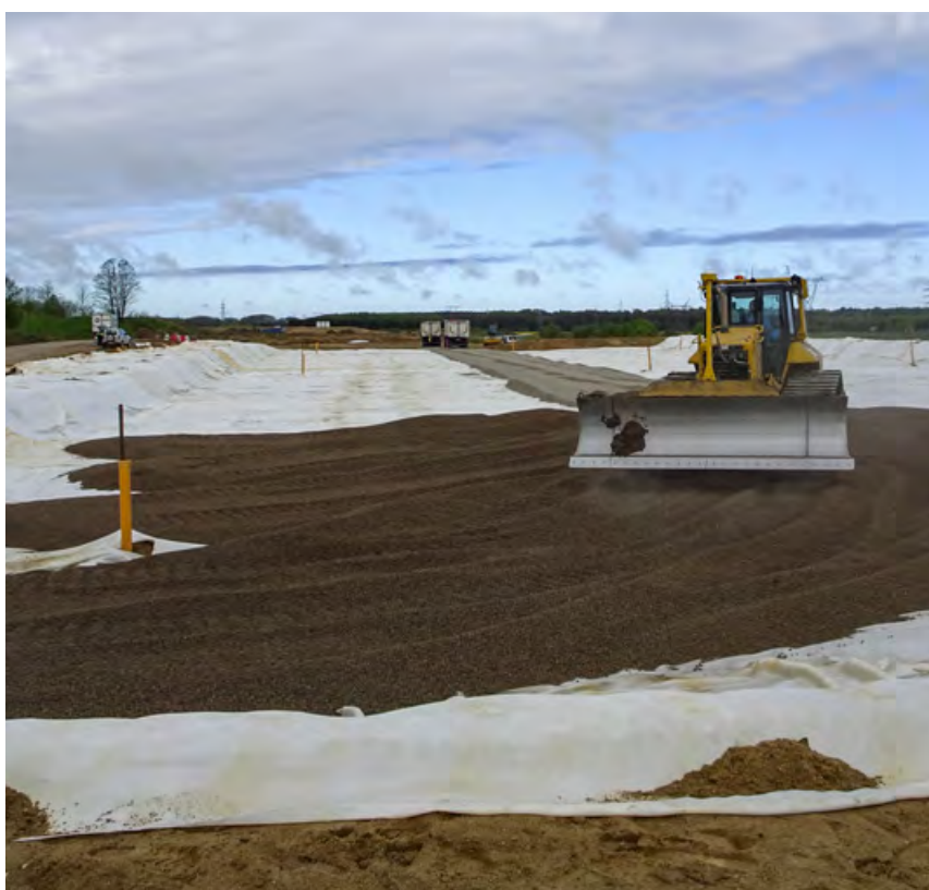
On three sections of the main route, mattress layers of Leca LWA (Leca® GEOTECHNICAL 8/10-20 RX) were designed and constructed
