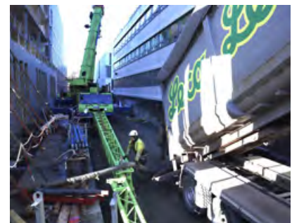
Cramped conditions on the construction site are no obstacle when the filler can be blown into place with long hoses (Photo: Jan Vestre)
