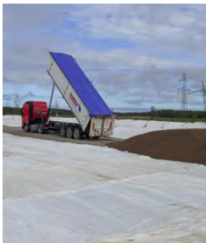
The work, which was originally carried out, was interrupted due to the considerable difficulties encountered due to the complicated hydrogeological conditions
