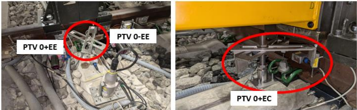
Figure 84.- Detail of the potentiometers used to measure the vertical displacements of the under-rail pad
