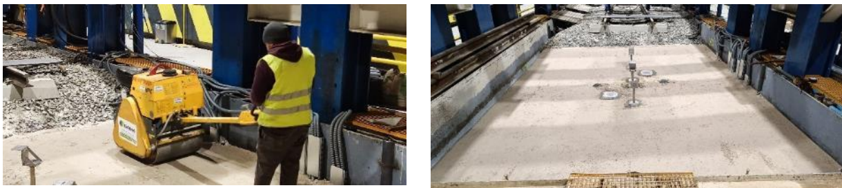
Figure 40.- Sub-ballast layer; left: new compaction machine, right: final aspect of sub-ballast layer
