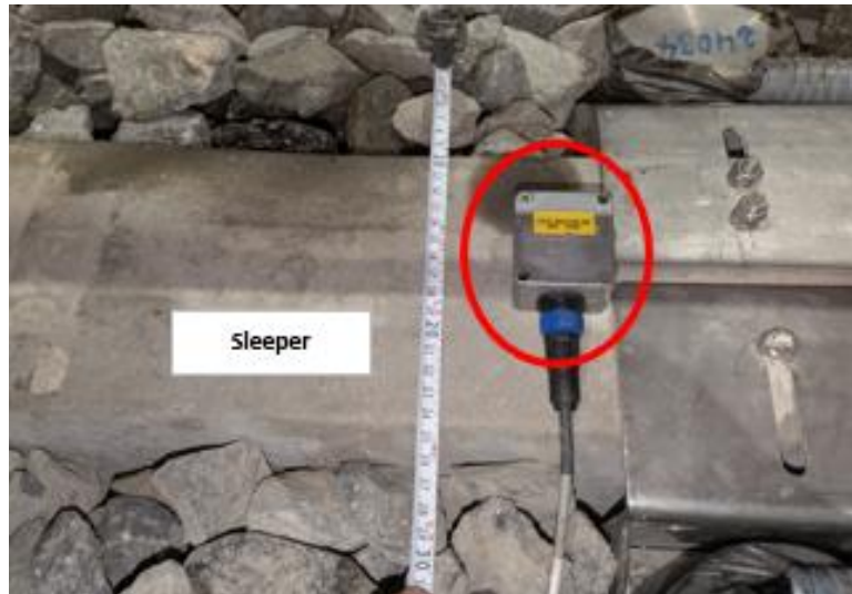
Figure 56.-Example of accelerometer located at sleeper
